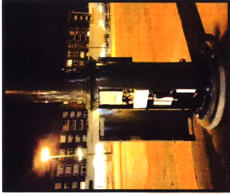
Equipment Inside of Pole Base
